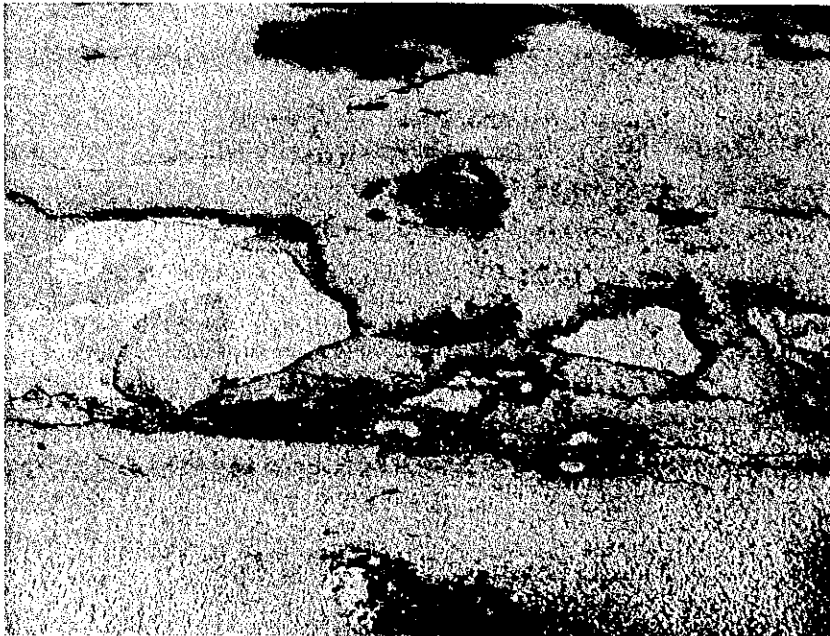
Potholes on Olden Rd.
