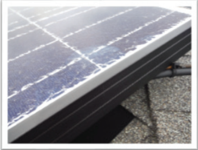
Photo D4: Equipment visibly damaged
